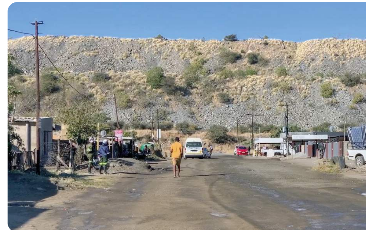
Damaged homes in Mmaditlhokwa and unsafe living conditions due to mining operations. Screenshot from North West Video , produced by Corruption Watch.
